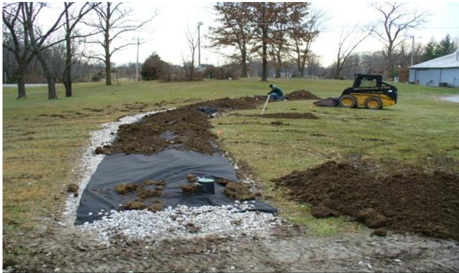
An at-grade system under construction. Notice the geotextile fabric covering the rock media.
